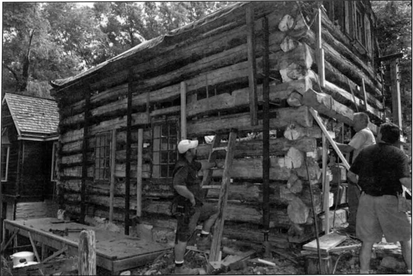
This image, taken July 25, 2008, shows Mr. Earle Marshall (second from right) and members of his team preparing to replace a weakened original log on the Church Road Cabin with a sound replacement, while doing no damage to the remainder of the structure. It is the full-scale equivalent of the child's game of Pick-Up Sticks , with catastrophic potential if done incorrectly. Courtesy of Roger D. Thorne.
